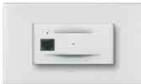
Wi-Fi access point
